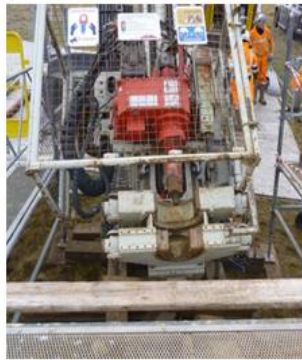
Angle of machine increases gap to working platform to an unacceptable distance.
