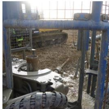
Large, unnecessary gap that permits access to dangerous parts.
