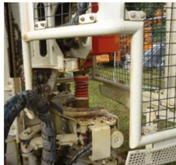
Large, unnecessary gap that permits access to dangerous parts.
