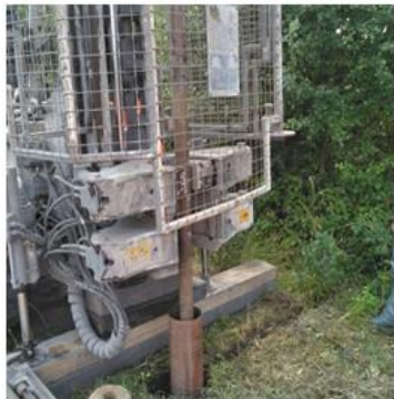
Guard starts too high from floor, doesn't prevent access to dangerous parts.
