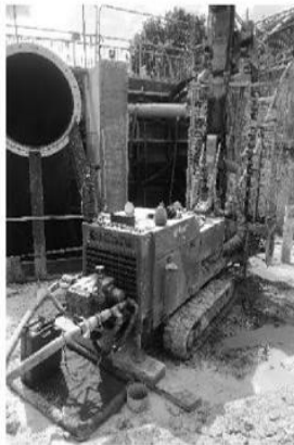
Rig following the incident
