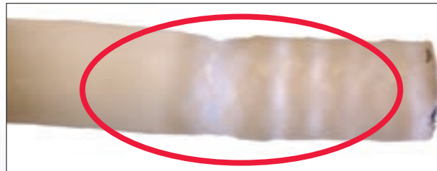
The above photograph shows a thinning of the liner such that leakage occurred
