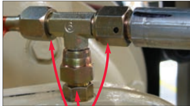
Checking that each elbow and T Piece remains firmly positioned and that there are no leaks around the port threaded interface and cone sealing areas.
