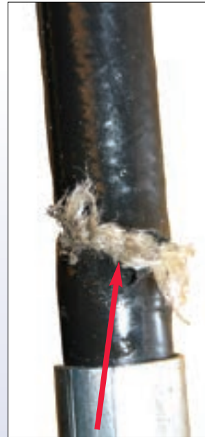
Hose burst near the ferrule
