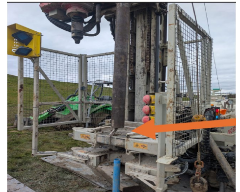
Photo 1: Arrow pointing to crush zone.
